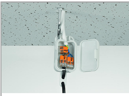
Pendant light connection in suspended ceilings
